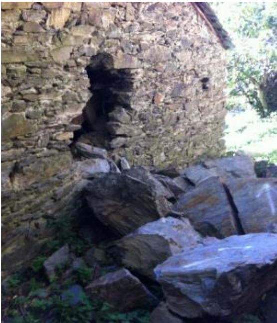
Fig. 9 The rockfall at Pont de Gullerí and the breach on the stone wall
