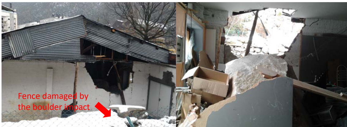
Fig. 11 Damage caused at a workshop in Andorra. Outside (left) and inside (right) view of the workshop
