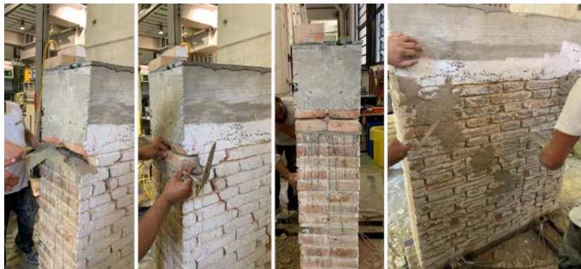
Figure 1: Scuci-cuci intervention on the URM tested walls. Removing and replacing of fractured units. Filling of cracks with lime-based mortar for repair.
