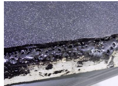
Figure 7. Increase in viscosity (melting) and microbubbles in the asphalt cement between the bituminous sheet and substrate.
