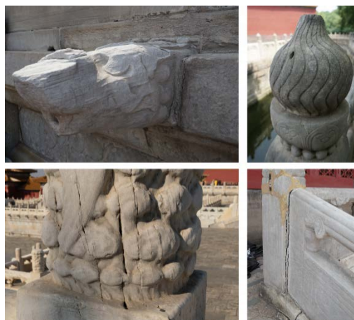
Figure 2. Mostly disease type of stone components(Top left: weathering; Upper right: scaling; Lower right: crack ; Lower right: shifting).
