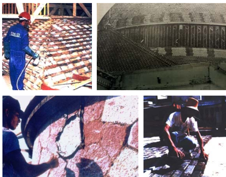
Figure 10: Amazonas Theater under renovation of 1987-1990: a) Treatment of the wooden structure of the Concert Hall plafond [18]; b) The dome roof [19]; c) Apparent surrounding wall restoration [18], d) The parallelepiped blocks restoration [18].
