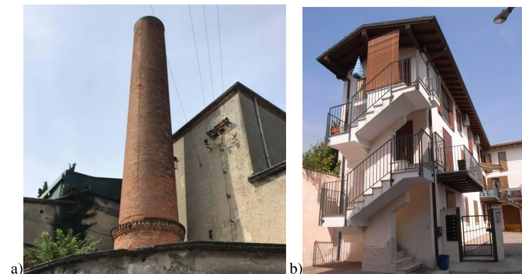
Figure 4: Fragilities in the structural units: a) slender elements; b) elements protruding on the road.
