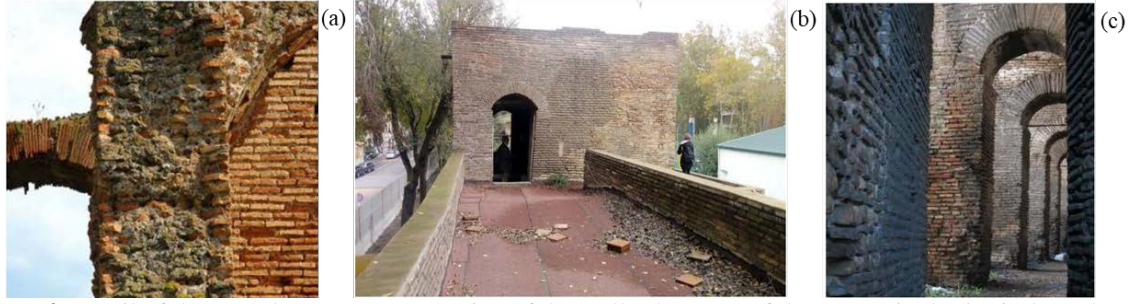
Figure 4: Detail of the opus latericium (a), portion of the walls close one of the towers in the b8-b9 branch (a) and transversal arches in the b9-b10 branch (b).
