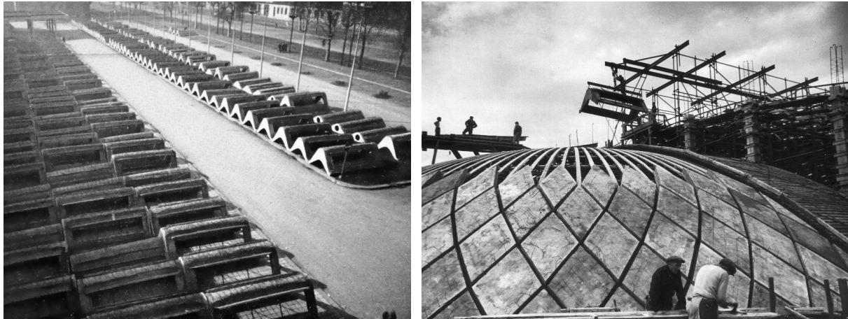
Figure 2: The onsite prefabrication procedure of the undulated ferrocement elements of Hall B and their positioning.
