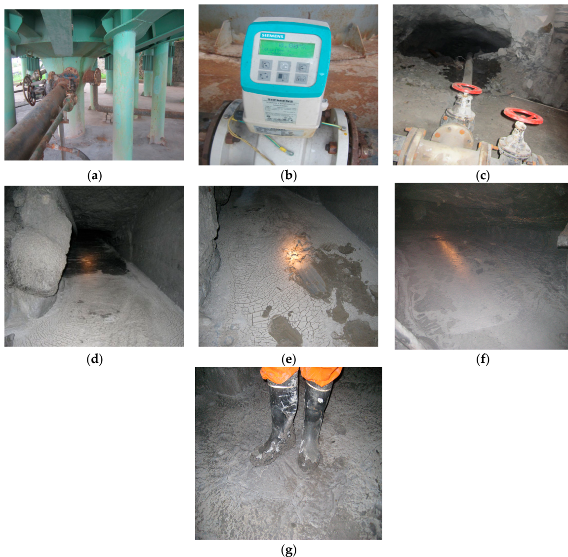
Figure 15. Backfilling transportation industrial test. (a) Thickener; (b) Electromagnetic flowmeter; (c) Pipeline transportation; (d) 24 h after filled (concentration 55%); (e) 72 h after filled (concentration 55%); (f) 24 h after filled (concentration 60%); (g) 72 h after filled (concentration 60%).
