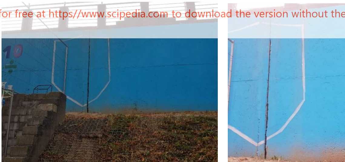
Figure 2. Two concrete slabs displaced due to ground washing.
