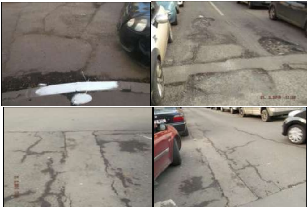
Figure 6. Degradation of the urban road structures
