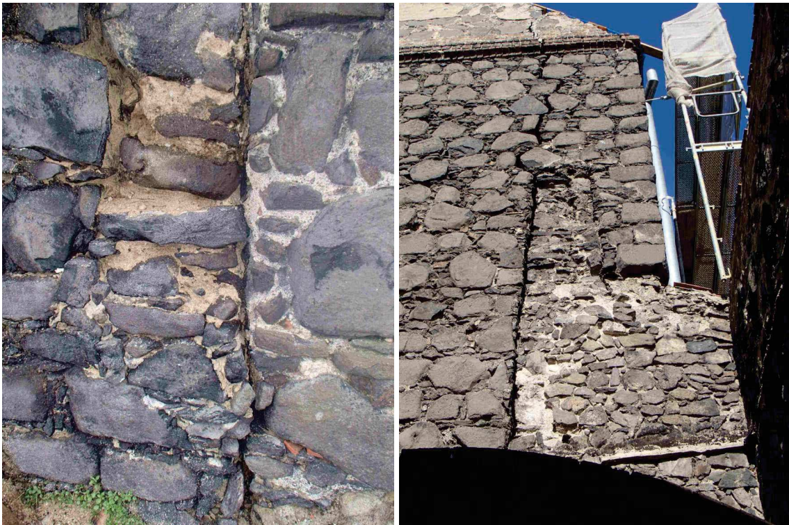
Figure 6: Exterior of the end walls with cracks along the external face of the defense wall
