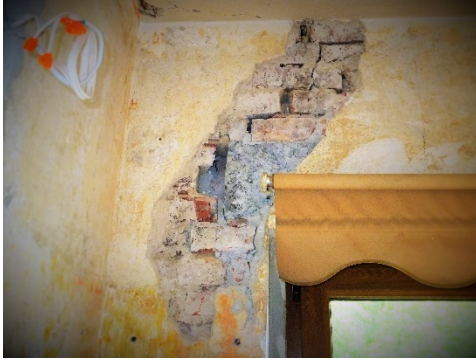
Figure 2. Cracks formed in a residential building in post-mining areas, around Bytom in Poland, 22/05/2011.
