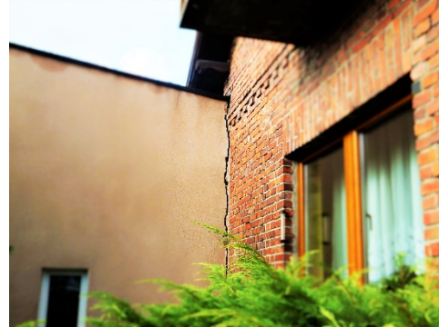
Figure 3. The uncontrolled dilatation of the building was created as a result of post-mining burst, around Bytom, 22/05/2011.
