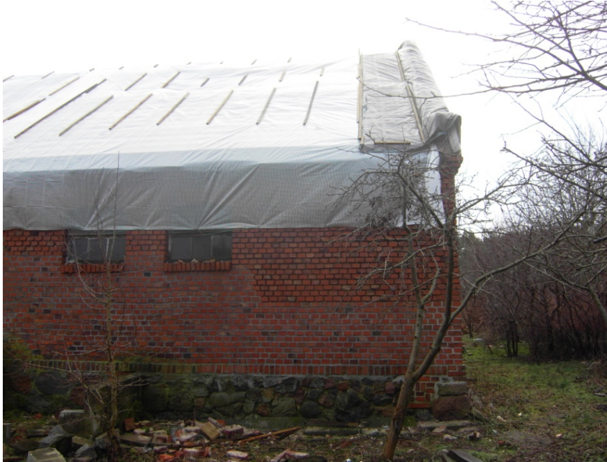
Fig. 5 The north wall of the outbuilding section with partial improper restoration with cement-lime mortar of the brick wall and cement of the stone plinth
