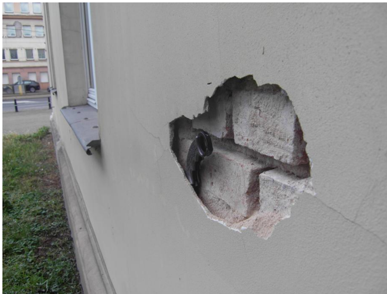
Fig. 3 Plaster on an exterior wall 15 years after renovation. It shows the complete destruction of the lime mortar covered by a too-tight and too-strong repair system from one of the leading companies in the local market
