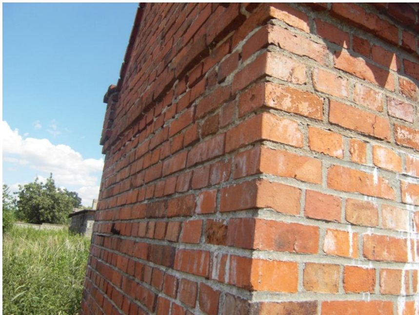
Fig. 6 The southwest corner of the farm section showing the good condition of the brick improperly jointed with cement-lime mortar. Still without damage caused by improperly applied material
