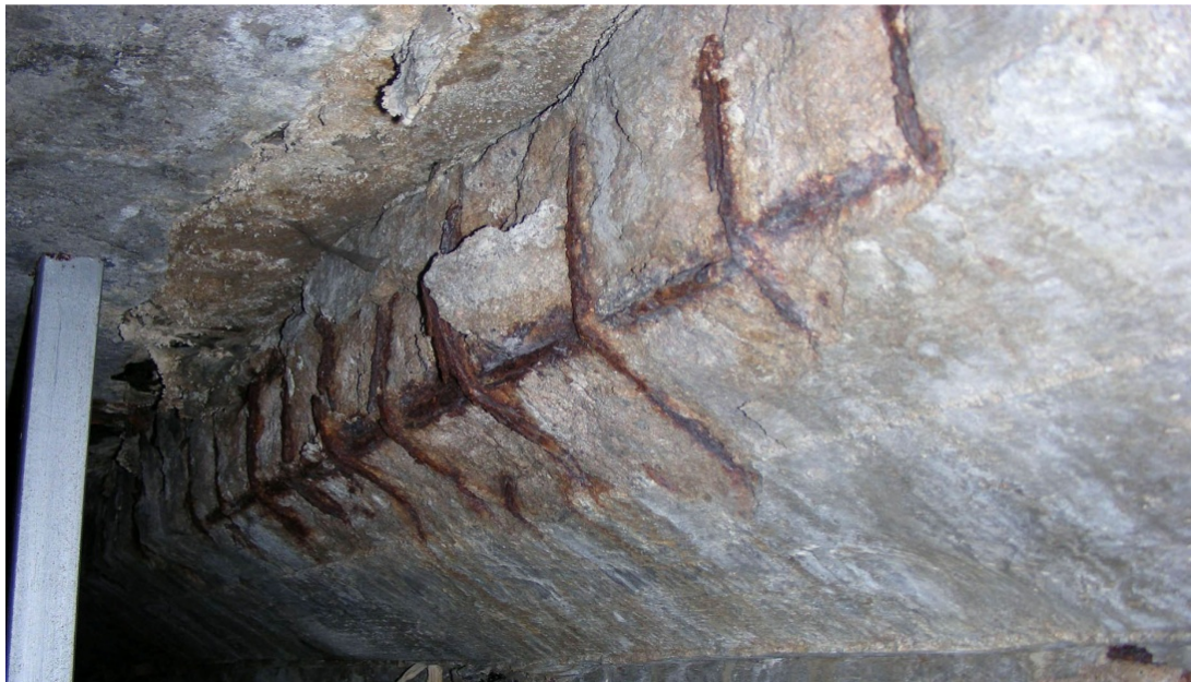
Fig. 7 Condition of the pool basin. Complete destruction of reinforcement, effect of carbonation of concrete
