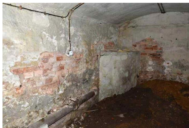
Figure 10: High dampness of the basement walls
