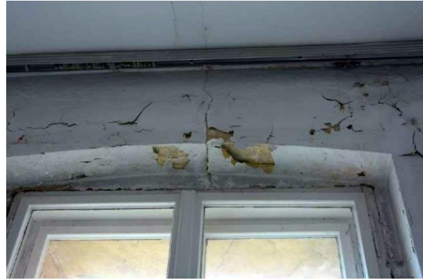
Figure 13: Exemplary cracks in lintels
