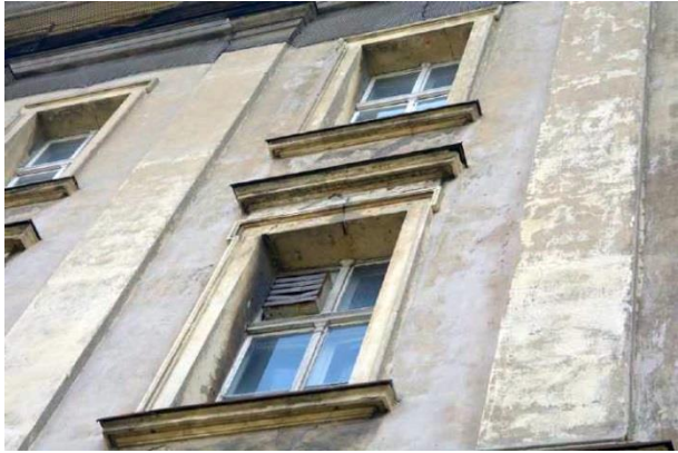
Figure 12: Example of cracks in lintels and walls
