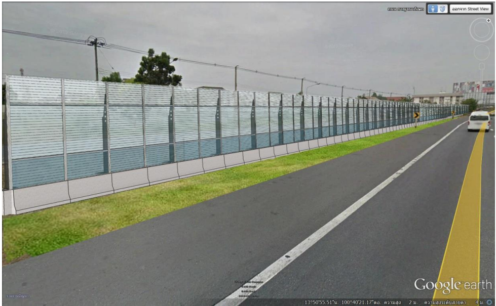
Figure 3. Noise Barrier on the Pilot Area
