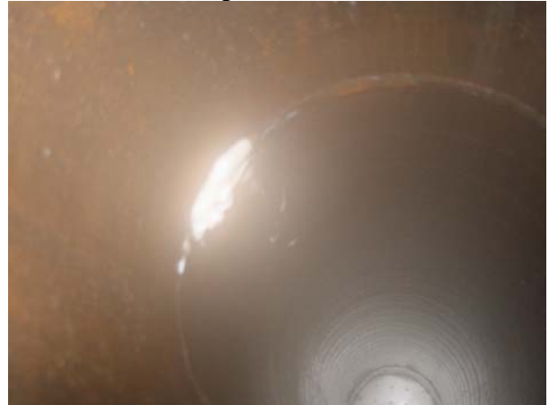
Photo 21: Soft Sealant Lump
