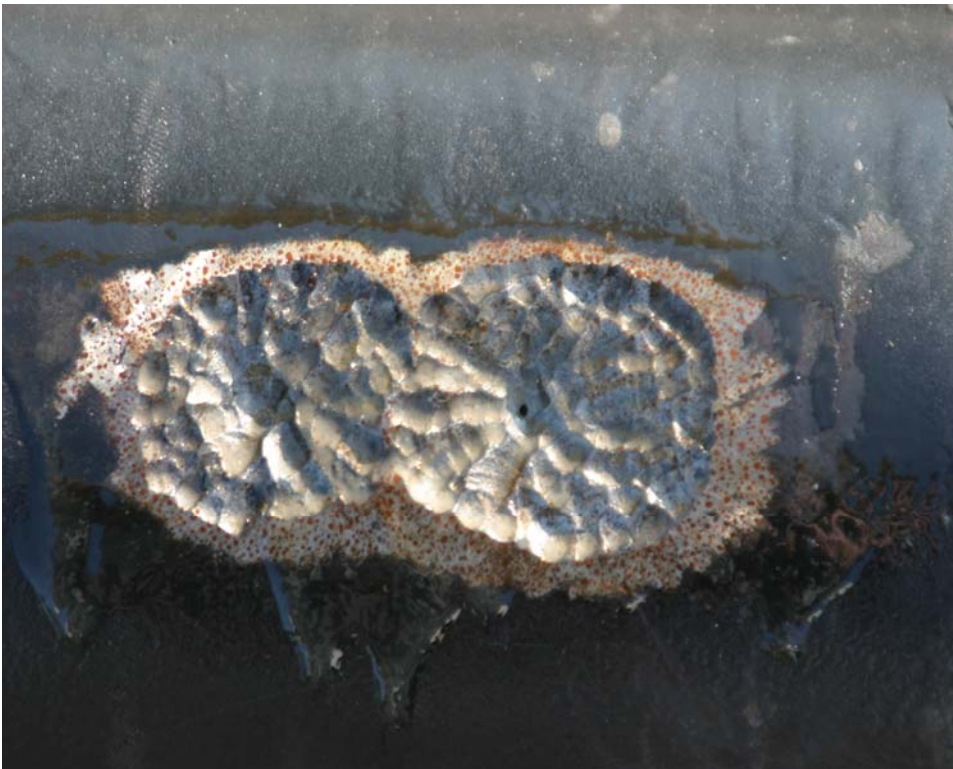
Photo 2: External Corrosion Defect
