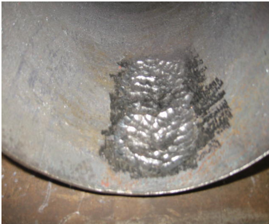
Photo 25: Internal Corrosion Defect - Bare
