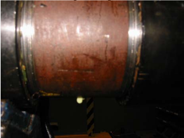
Photo 31: Sealant Extruding Through Pinhole
