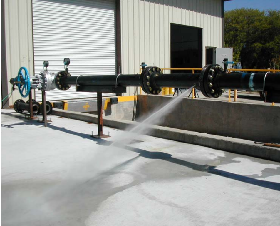
Photo 8: Internal Corrosion Leak Rate Testing
