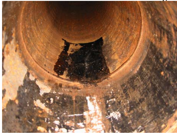
Photo 26: Internal Corrosion Defect with Flex-Plug
