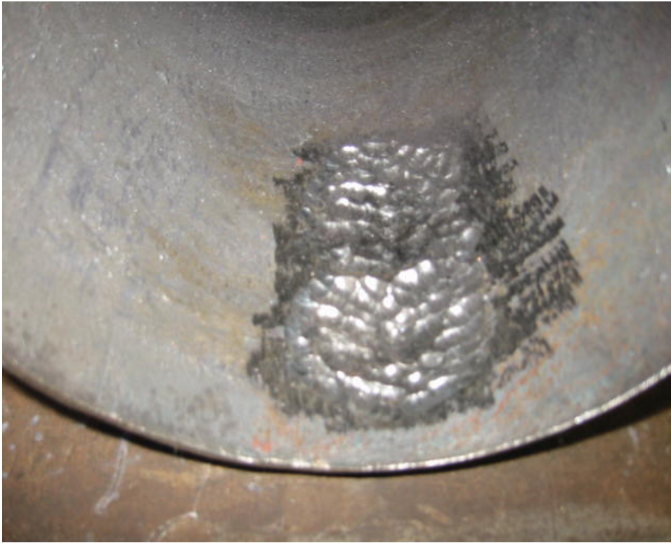
Photo 3: Internal Corrosion Defect
