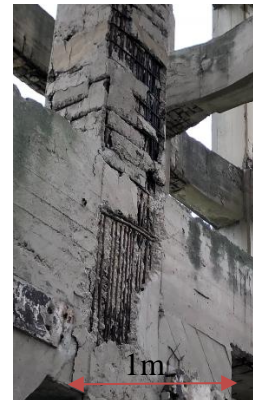
Figure 4. Rebar exposure due to spalling.
