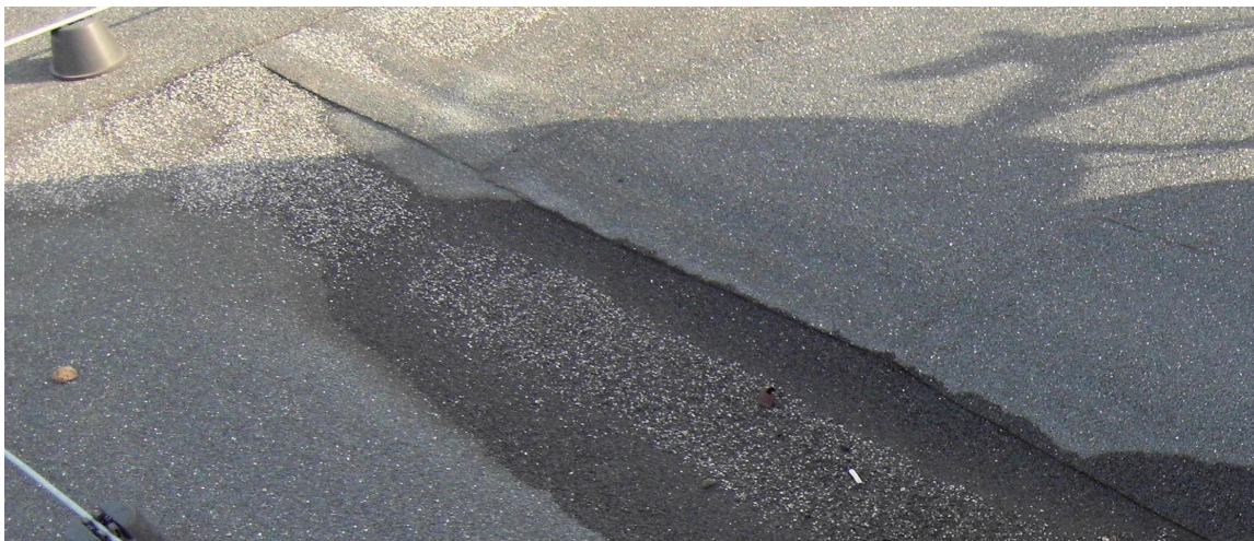
Figure 5. Accumulation of released granules (roof after one year of operation)
