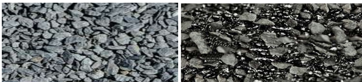
Figure.1 This is a comparison of mineral topping on new roofing paper and topping on the same roofing paper after several years of use in adverse conditions (on the right photo a drastic example of a significant loss of granules and exposure of asphalt in a roof depression - a periodic puddle).
