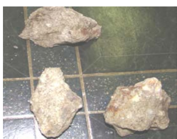
Figure 9. Pieces of Concrete B; completely carbonized concrete (all the way to the reinforcement bars) with visible remains of corroded reinforcement ( \text{pH} > 9 ).
