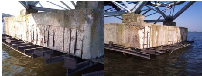
Figure 1, 2. Damages to pillars in the form of spalling corroded concrete and corroded reinforcing steel.
