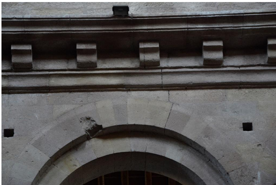
Figure 3: Lesions on the arches keystones along the nave wall.
