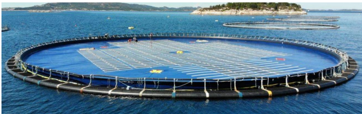
Figure 1 Floating photovoltaic power plant by Ocean Sun.
