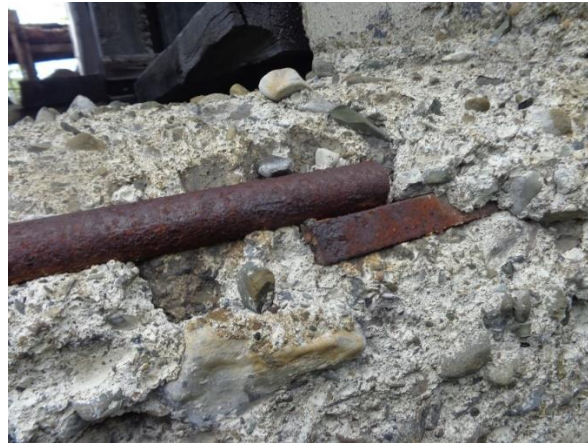
Figure 3: A round bar overlapped with a square bar in a splice. Also note variation in aggregate size and shape
