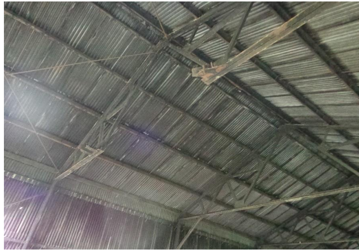
Figure 2: Roof truss with part of the bottom chord removed
