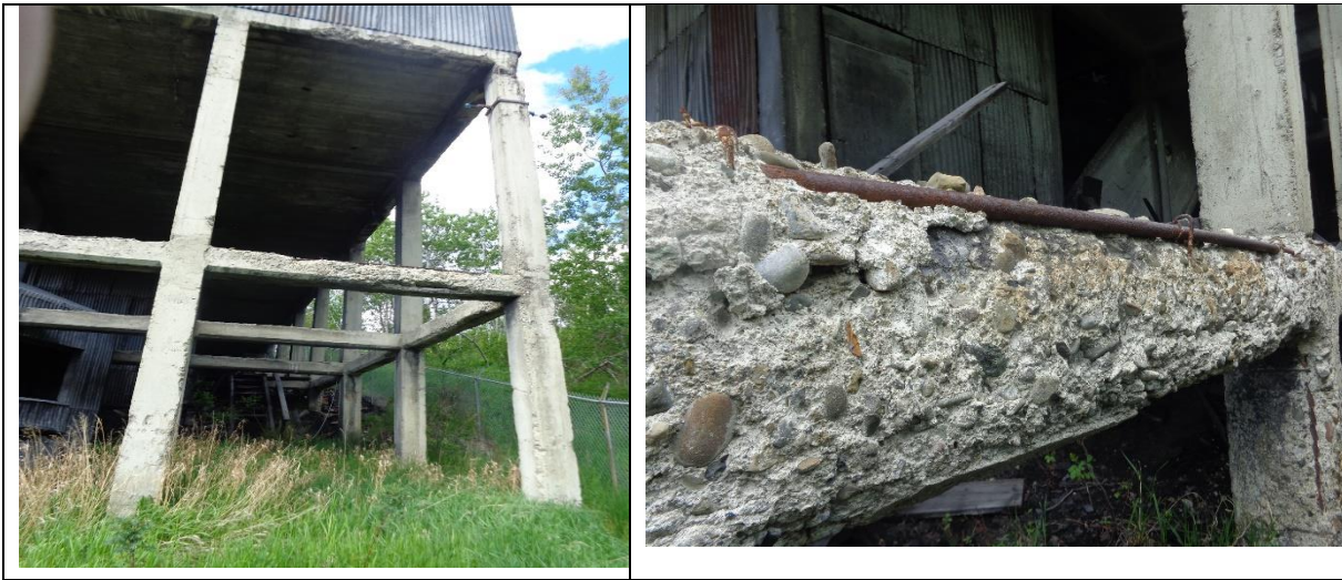
Figure 4: Signs of deterioration on concrete members
