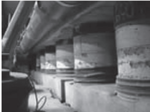
(a) Highly deformable concrete slots (Solexperts HDC®) in Chienberg tunnel (Jura Mountains).
